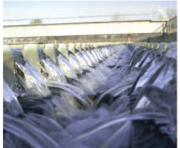
Indianapolis, Indiana Water Treatment Facility
